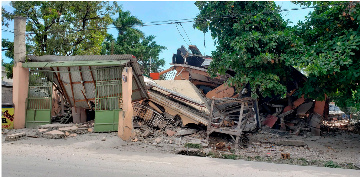
The Cayimite Hotel is damaged after an earthquake in Les Cayes, Haiti, Saturday, Aug. 14, 2021. (AP Photo/Delot Jean)
