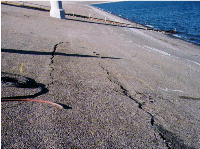
Surface cracks from 1994 quake
