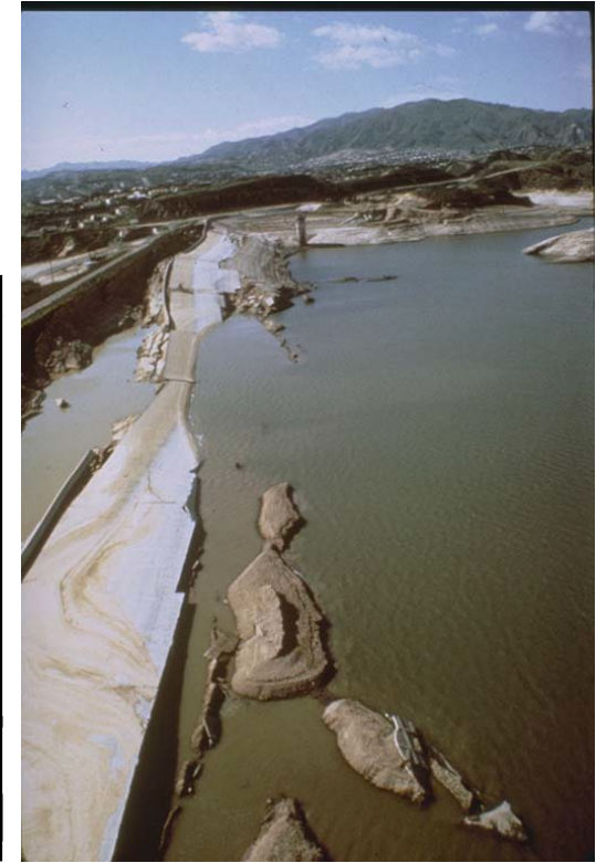
Dam failure from 1971 quake
