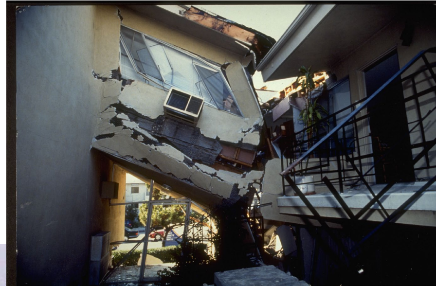
Sixteen people were killed when the Northridge Meadows apartment complex collapsed. Image courtesy of FEMA News Photo
