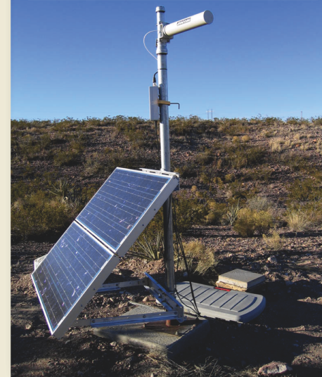
Station with radio communications solar power system
