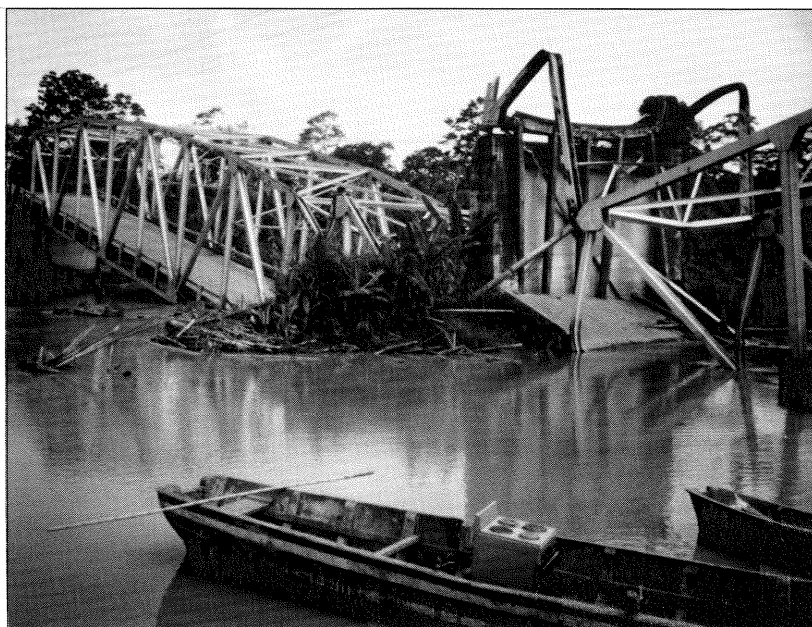
Figure 2. Photograph of a collapsed bridge on the road between Limon and Cahuita, Costa Rica.
